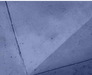
Carbonated building elements
